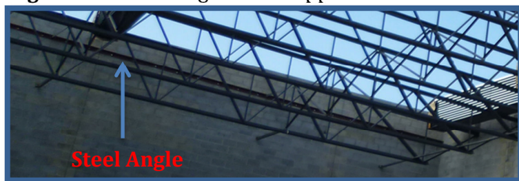
Figure 1.2: Steel Angle Deck Supports
